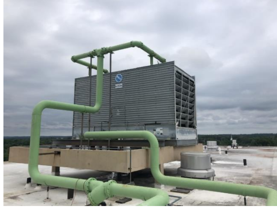
BAC 500 Ton Cooling Tower Estimated System Volume = 2,916 gallons Sump 8' X 16' / 480' of 10" Piping
