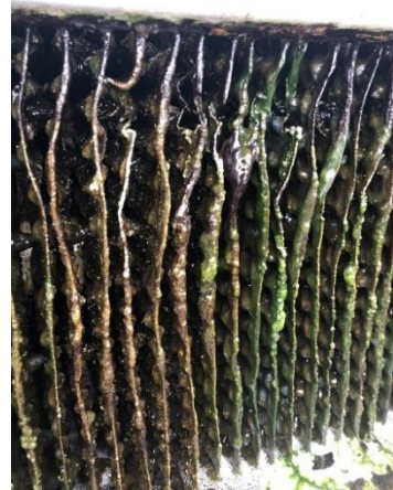
Tower Fill with Heavy Build-up
