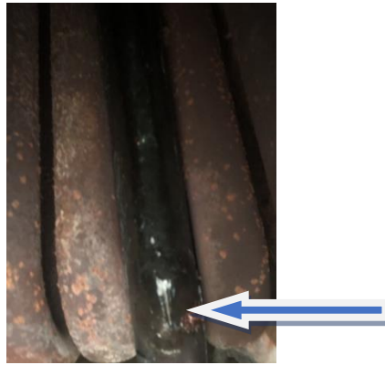
Leaking Tubes in Heat Loop
