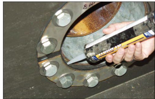
Figure 17. Caulk Exposed Galvanized Steel
