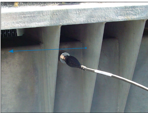
Figure 14a. Accelerometer Location - Gear Drive
